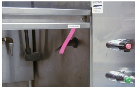
Figure 16. Air flow indicator.
